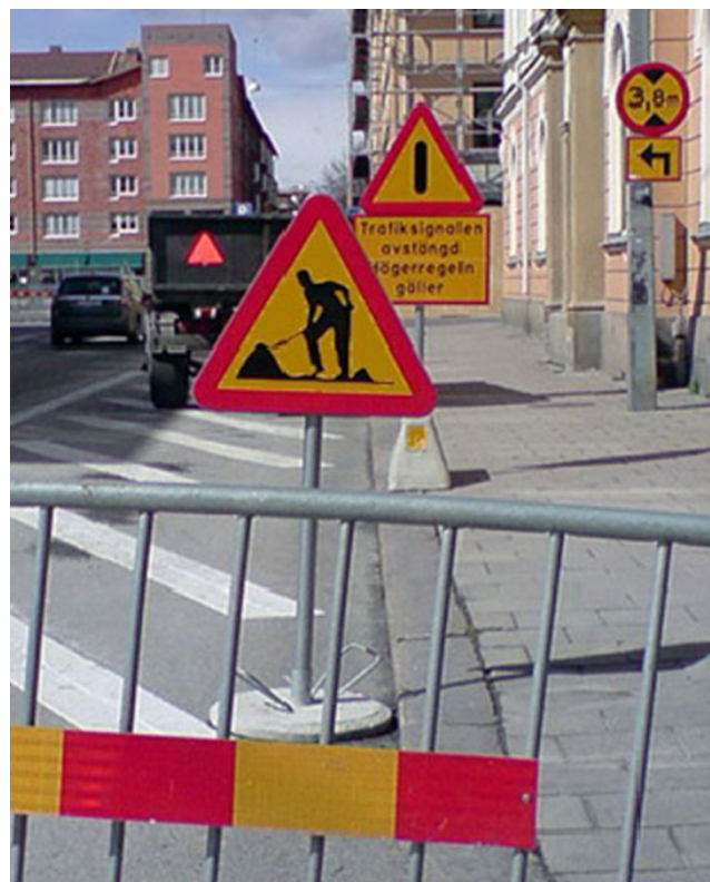
Fig. 2 Each traffic sign is in itself highly visible, but in this competitive environment the conspicuity of each sign is diminished by the other signs
