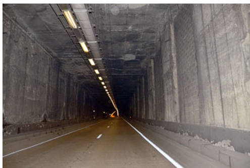
Fig. 9 Inside view of test site within Leopold II tunnel in Brussels, before renovation
